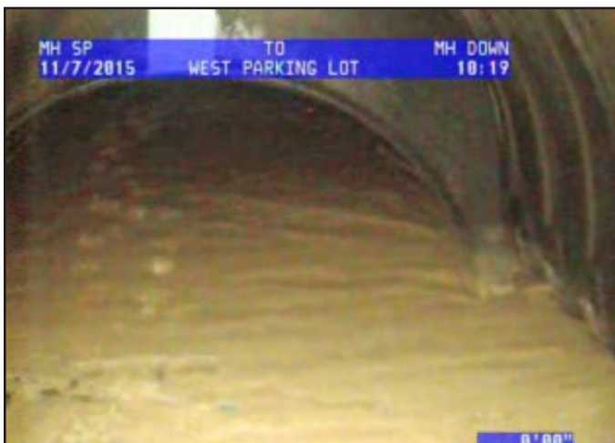
SEPARATOR ROW: Separator Row prior to cleaning
