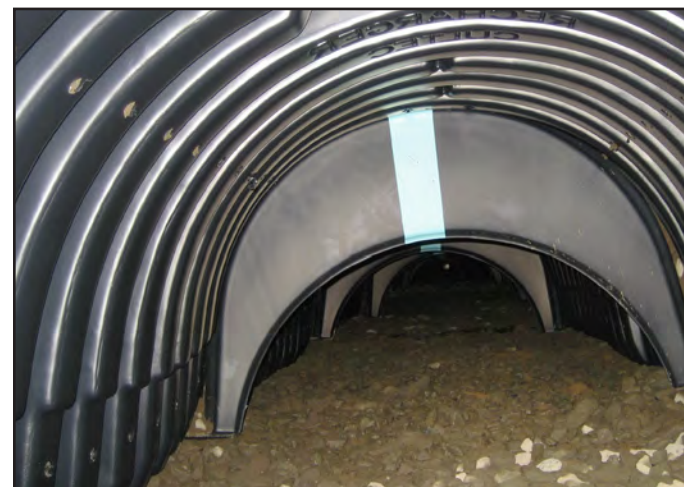
ADJACENT ROW: When the Separator Row is working properly, the adjacent rows will not show signs of sediment.
