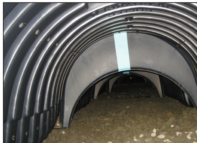
ADJACENT ROW: When the Separator Row is working properly, the adjacent rows will not show signs of sediment.
