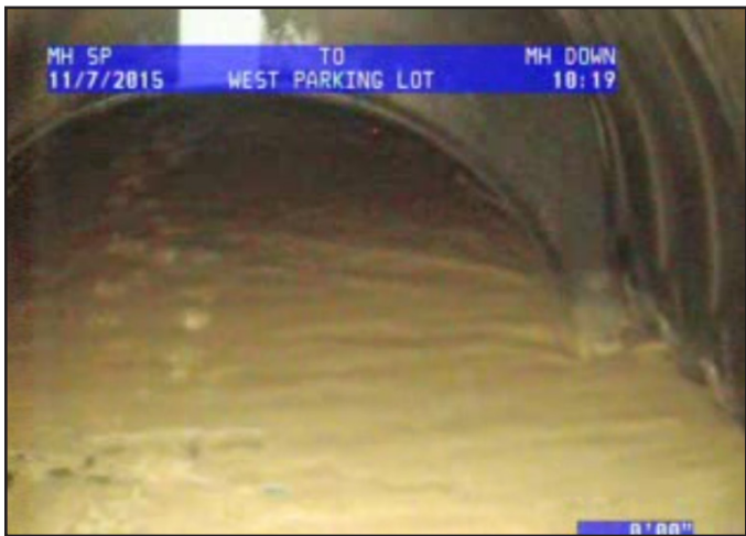
SEPARATOR ROW: Separator Row prior to cleaning
