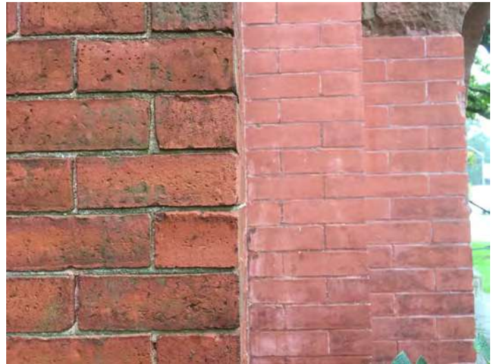
Fig. 6: Inappropriate brick replacement
