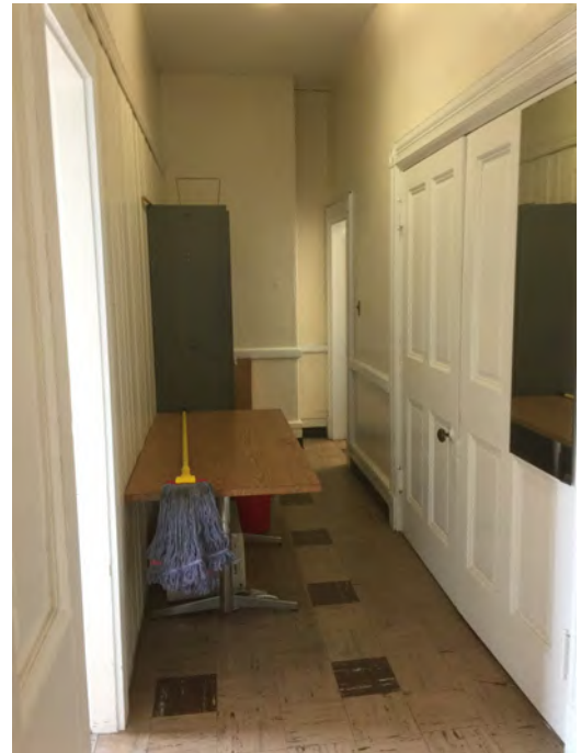
Fig. 10: Potential asbestos floor tile
