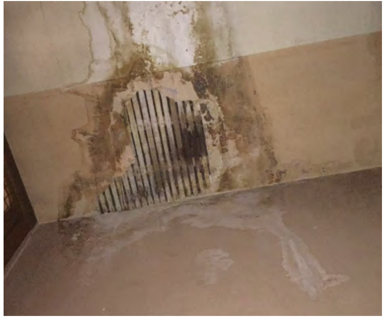
Fig. 2: Roof leak, failing plaster + damaged finishes
