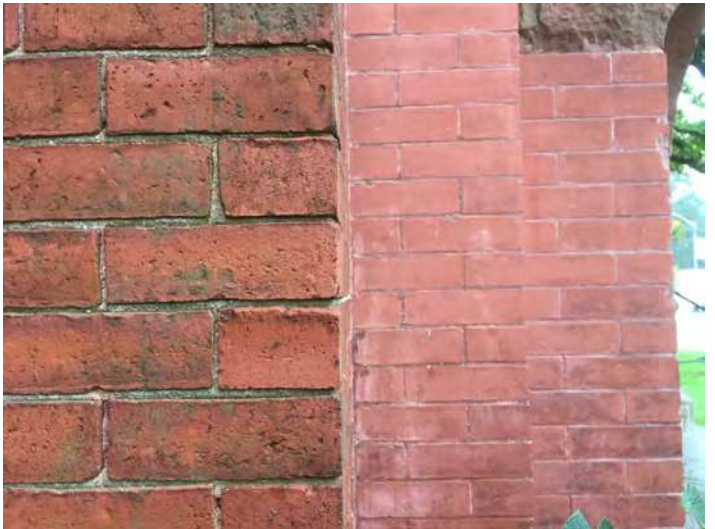
Fig. 6: Inappropriate brick replacement
