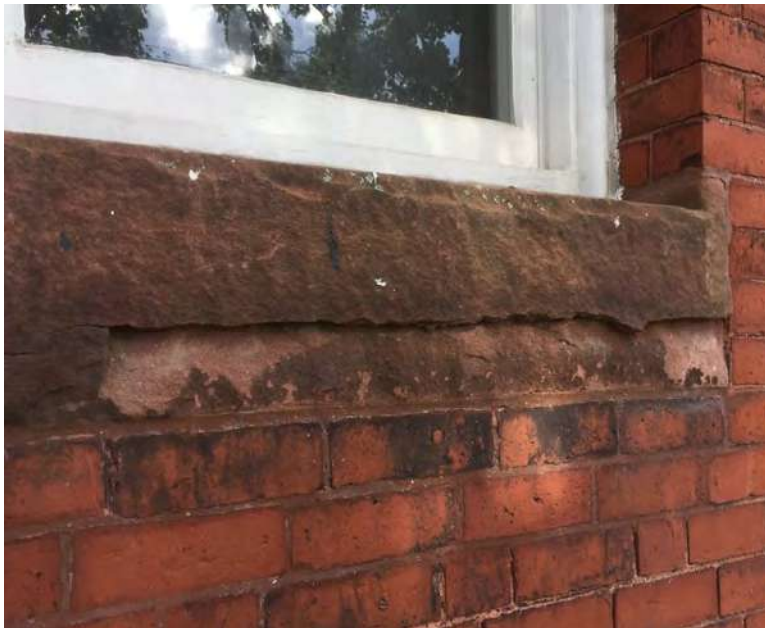
Fig. 5: Spalling brownstone sill
