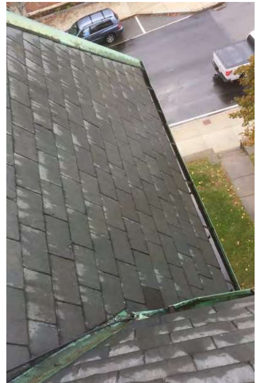
Fig. 4: Clogged and damaged gutter and valley flashing
