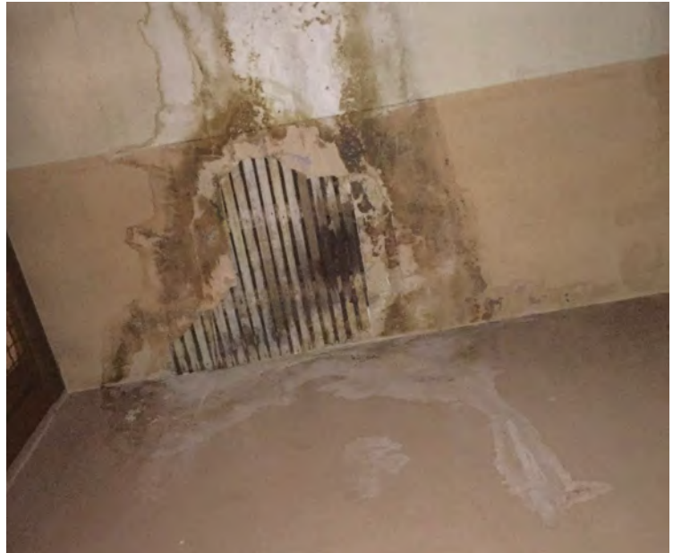
Fig. 2: Roof leak, failing plaster + damaged finishes
