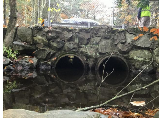
Figure 15. View of existing crossing outlet on Smith Avenue (xy42165037124747) taken during field assessment on October 29, 2019.
