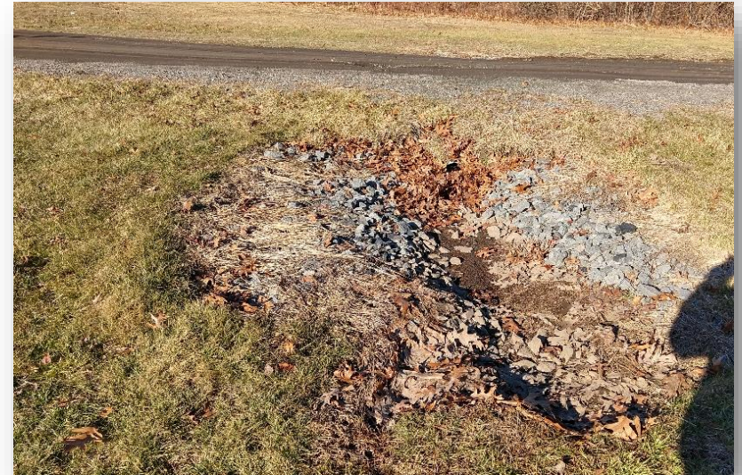
Image 1: Existing stormwater outfall (partially obscured by leaves).
