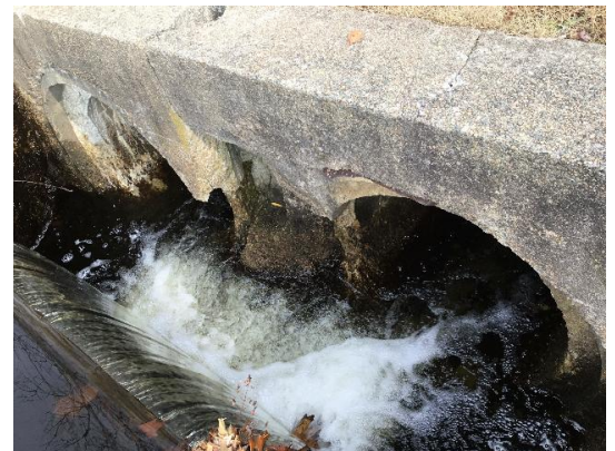
Figure 25. View of existing crossing inlet (xy42138987124132) taken during field assessment on November 11, 2019.
