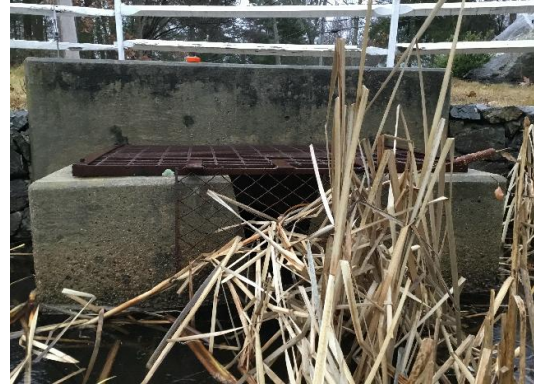
Figure 22. View of existing inlet on Audubon Drive (xy42134647125771) taken during field assessment on November 22, 2019.
