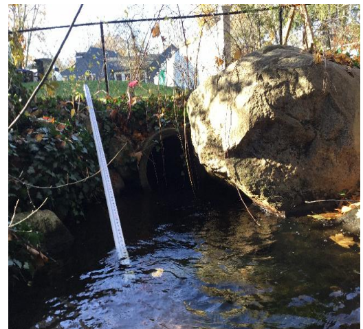
Figure 20. View of existing outlet on Spring Valley Drive crossing (xy42137957125730) taken during field assessment on November 6, 2019.
