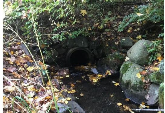
Figure 34. View of existing crossing inlet taken during field assessment.
