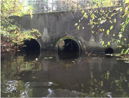
Figure 14. View of existing crossing outlet on Gould Street (xy42165167124759) taken during field assessment on October 29, 2019.
