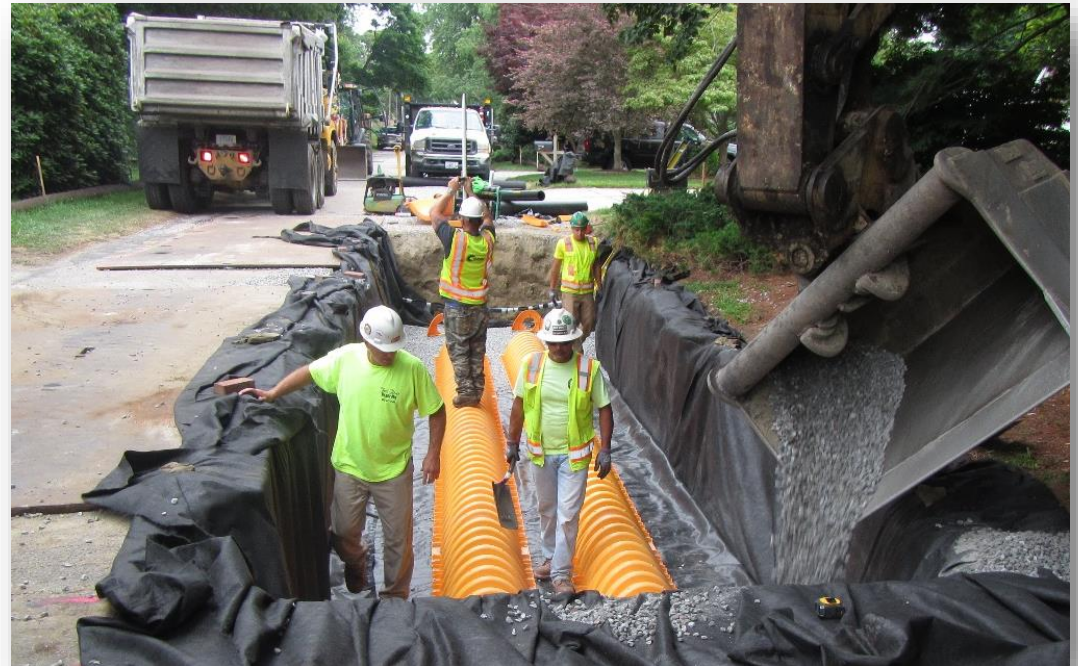
Image 1: Installation of subsurface infiltration chambers under one lane of a municipal right-of-way in Rhode Island.
