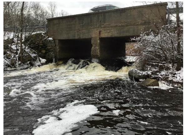
Figure 23. View of existing box culvert outlet taken during field assessment on December 13, 2019.
