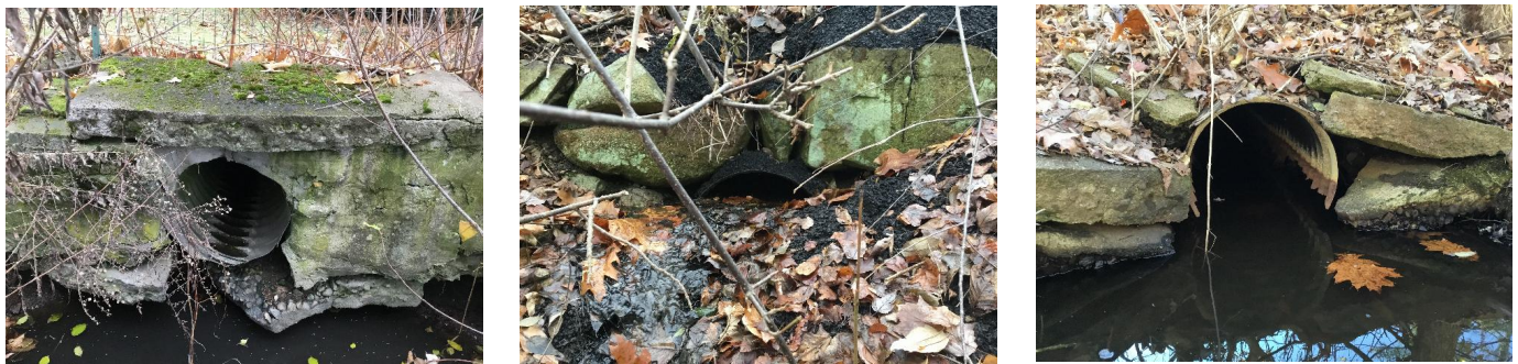
Figure 3. Examples of crossing structures in poor or critical structural condition observed at various locations during field assessments. Left: Degraded headwall; Center: Critical level of blockage; Right: Deteriorated pipe invert.
