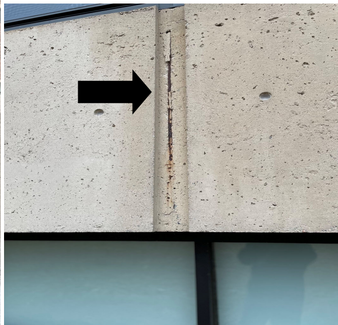
Typical exposed rebar and spalling concrete
