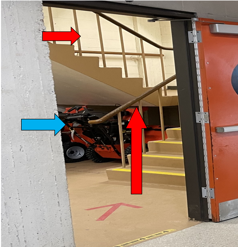
Arrows identify baluster spacing non-compliant with MSBC & Handrails to compliant with MAAB. Blue arrow demonstrates operational need to relocate gas powered equipment to a proper storage area.
