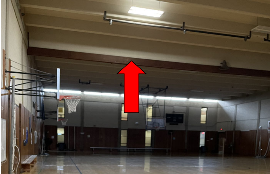
Location of non functional gym wall
