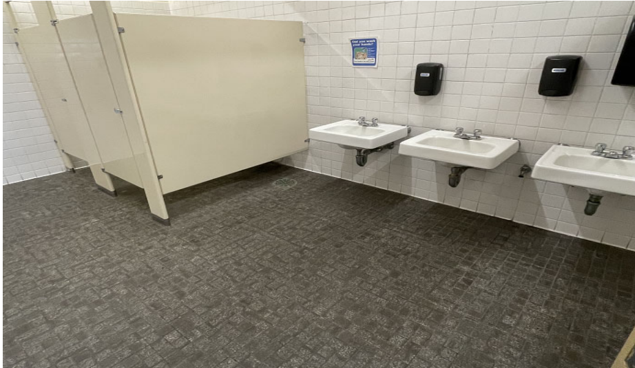
Typical existing bathroom lacking handicap assessable fixtures
