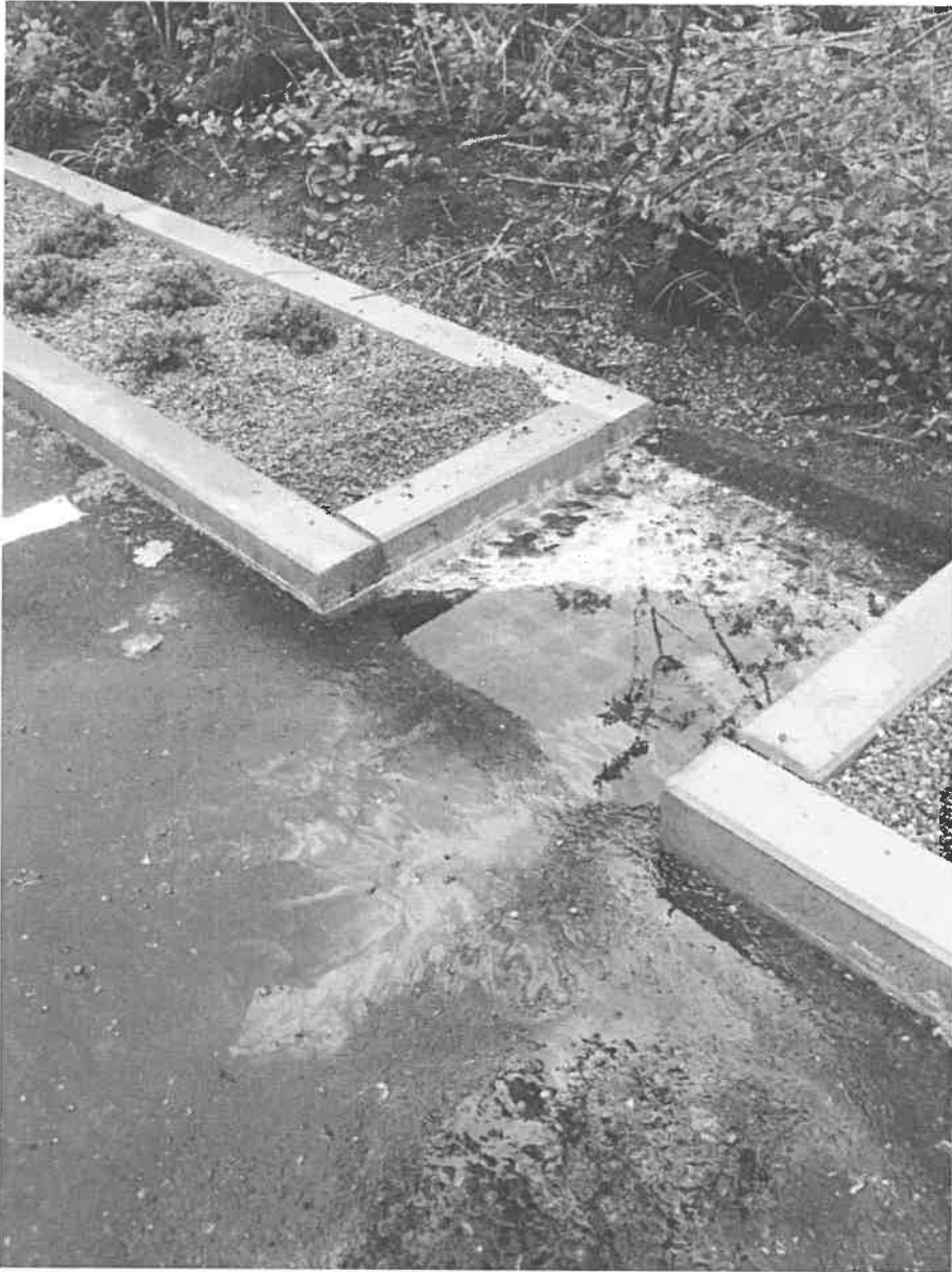
Figure 2 – Hydrocarbon sheen on stormwater entering stormwater system.
