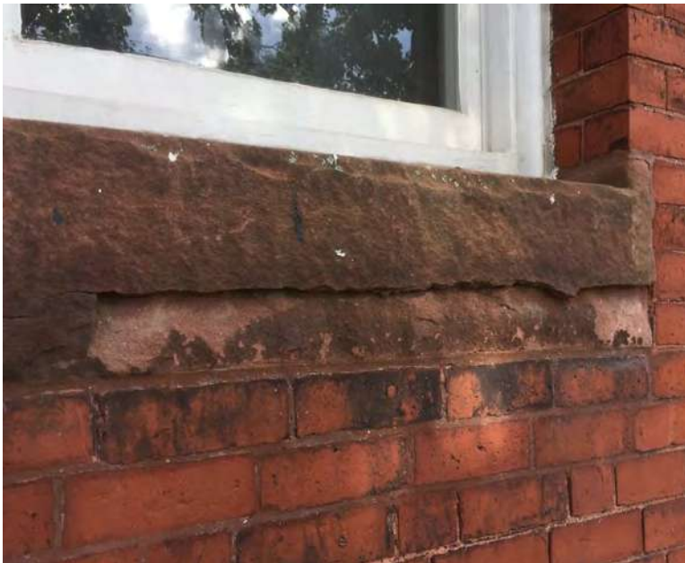
Fig. 5: Spalling brownstone sill
