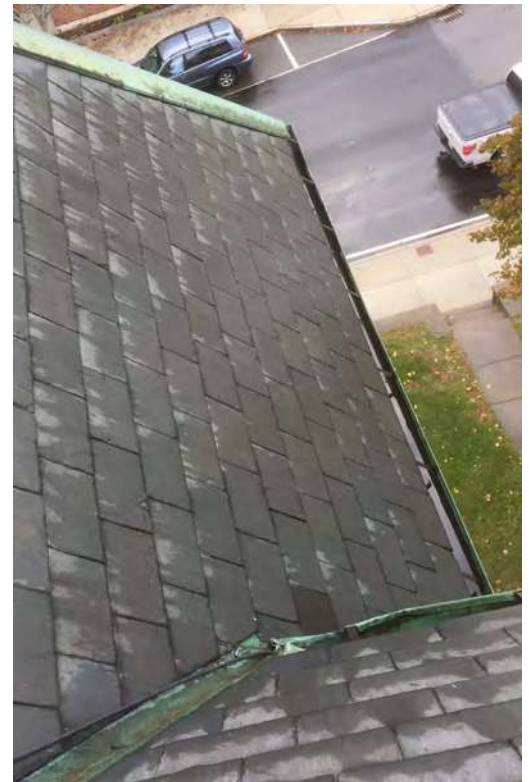
Fig. 4: Clogged and damaged gutter and valley flashing
