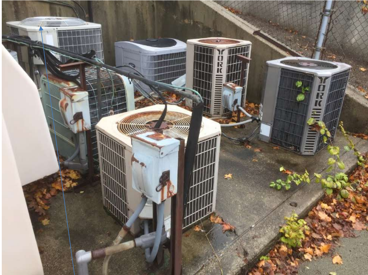
(4-ton condensing unit)
