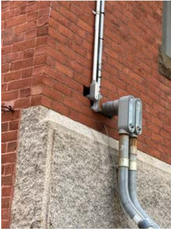
Unsealed wall penetrations
