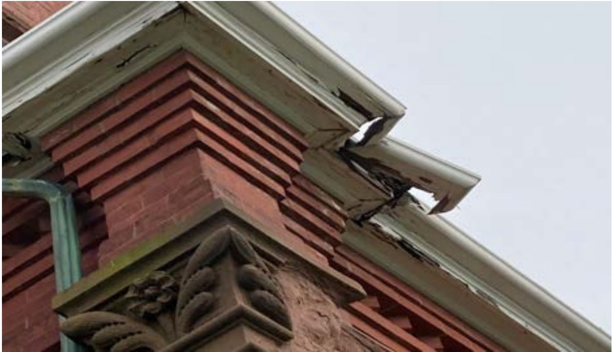
Front porch wood gutter failure
