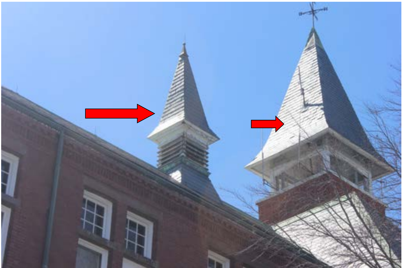
Broken and missing slate. Cupola trim rotted and open up at joints
