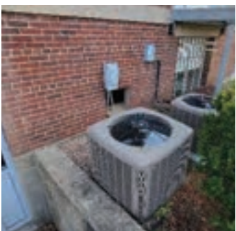
Photo 27: Outdoor CUs that serve the indoor ACs terminations
