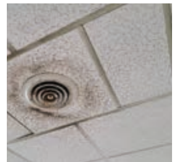
Photo 23: View of staining/mold at Level 1 recreation room ceiling
