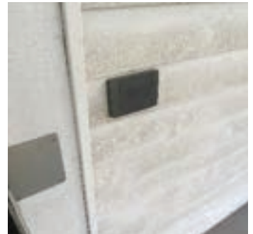
Photo 21: View of outdoor switch
