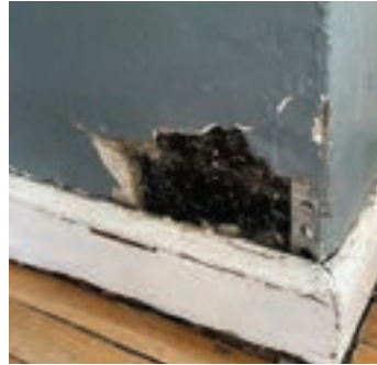
Photo 18: View of plaster damage in auditorium
