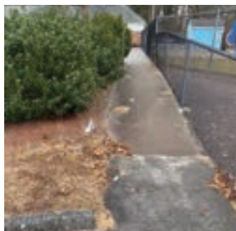
Photo 2: Overgrown planting and non-accessible walkway at parking lot
