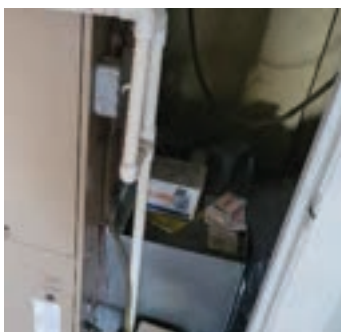
Photo 26: View of AC that serves the auditorium/gym
