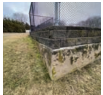
Photo 4: Drainage concerns at wall
