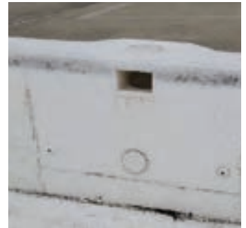
Photo 17: Center Pool skimmer
