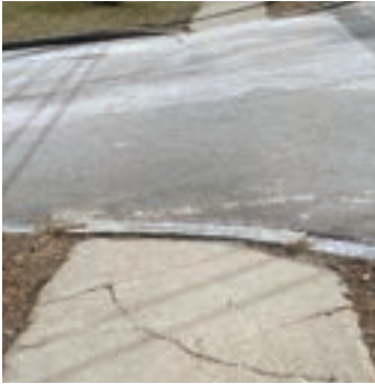
Photo 3: Non-compliant sidewalk crossing
