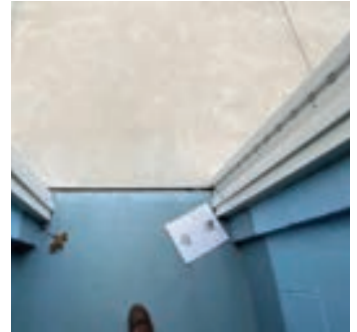
Photo 3: Gap at doorway
