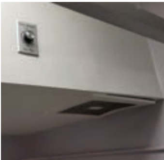
Photo 33: Typical bathroom exhaust fan
