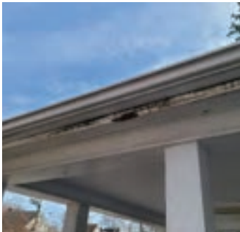
Photo 10: Damage at porch fascia boards
