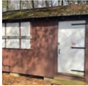
Photo 13: Moss growing on cabin roof
