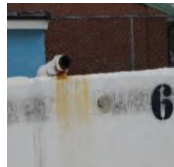
Photo 29: South Pool Autofill System
