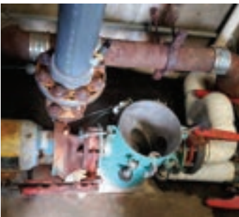
Photo 25: Corroded equipment, piping, valves and pipe supports
