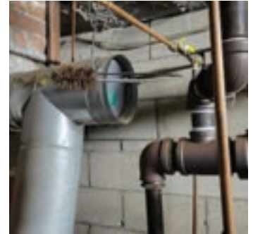
Photo 28: Boiler flues into the chimney
