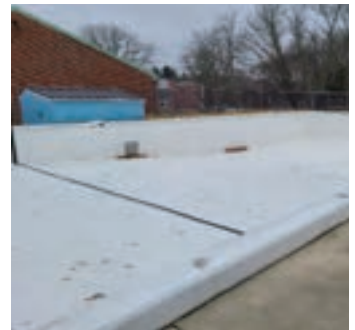
Pool and mechanical room, South Pool
