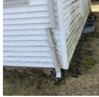
Photo 5: Damaged and inoperable downspout
