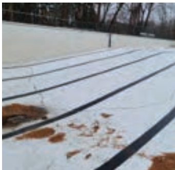
Photo 6: Cracks at deep end of Central Pool
