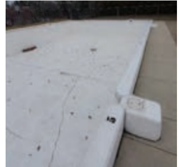
Photo 28: Cracks in pool
