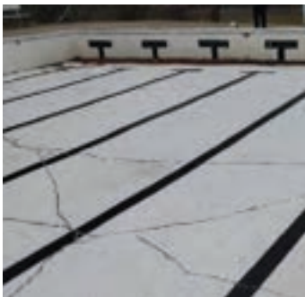
Photo 20: Cracking in Center Pool shell
