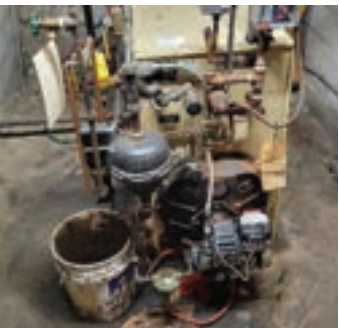
Photo 26: Existing Weil McLain boiler
