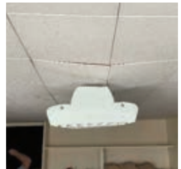
Photo 8: View of sagging ceiling in attic
