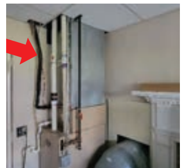
Photo 30: Combustion air split needs repair
