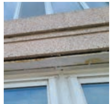
Photo 21: View of the rusted steel lintels over windows
