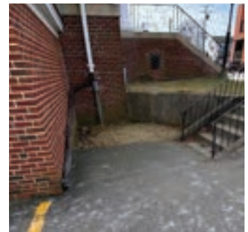
Photo 8: Site drainage issue at Northeast corner
