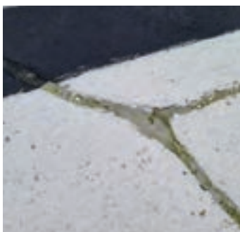
Photo 7: Large crack at the bottom of the Center Pool
