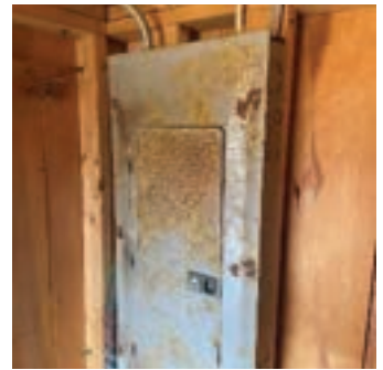
Photo 26: Rust and corrosion at panelboard
