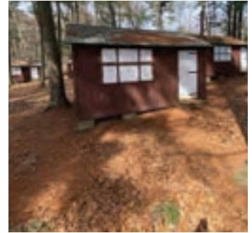
Photo 3: Minor erosion around cabins
