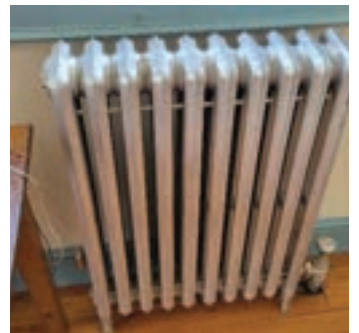
Photo 30: Typical cast-iron radiator
