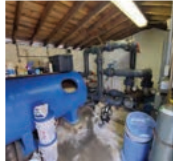
Mechanical room, South Pool
