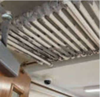
Photo 16: View of ceiling mounted radiator
