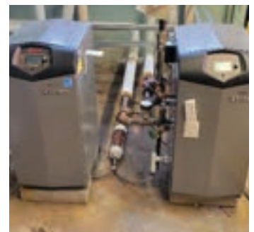
Photo 31: Existing lochinvar boilers
