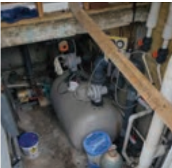
Photo 23: Wading Pool and splash pad equipment room
