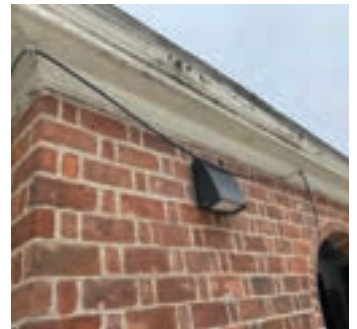
Communications and site lighting, Center Pool
