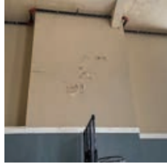
Photo 19: View of paint peeling around chimney
