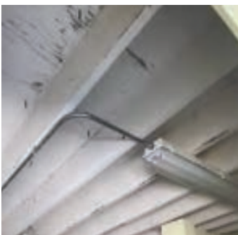
Photo 27: Interior fluorescent lighting
