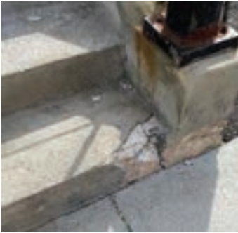
Photo 10: View of stairs cracking
