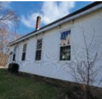
Photo 25: Windows provided ventilation air
