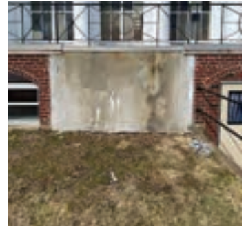
Photo 7: Site drainage issue at South facade
