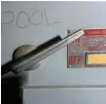
Photo 25: Main service disconnect at Boyden Elementary
