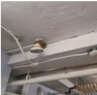
Photo 24: Cracks in level 1 men's bathroom concrete
