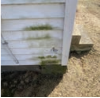
Photo 3: Drainage concerns at building foundation
