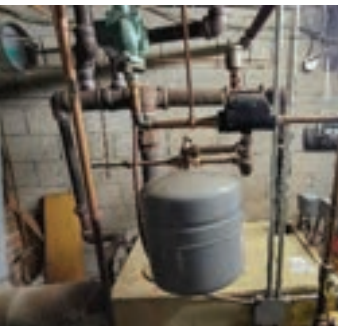
Photo 27: System pump and appurtenances
