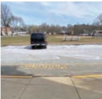
Photo 2: Non-compliant curb cut
