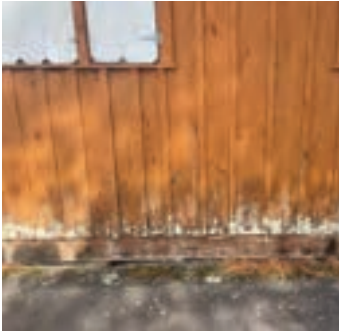
Photo 12: Mold and algae growth on siding
