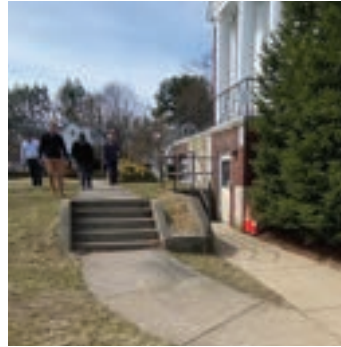
Photo 4: Non-compliant southeast stairs
