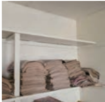
Photo 11: Cracks in attic space walls
