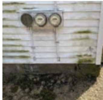
Photo 18: Siding mold damage
