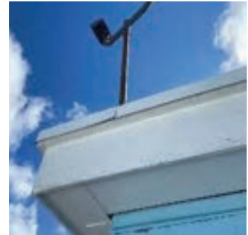
Photo 28: Current exterior lighting
