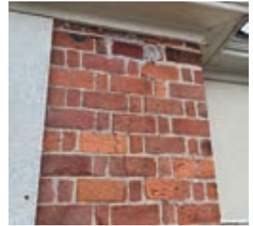
Photo 10: Rusted steel lintels inside building
