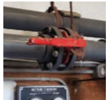
Photo 19: Center Pool pipe supports
