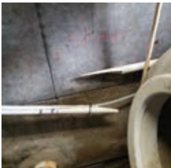
Photo 24: Broken feed pipe
