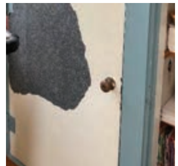
Photo 7: View of painting chipping on metal door
