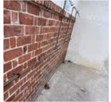
Photo 3: Erosion outside of pool deck
