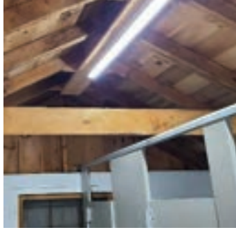
Photo 20: Mold and algae growth on siding
