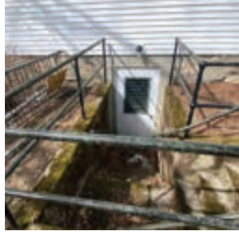
Photo 4: Drainage concerns at bulkhead
