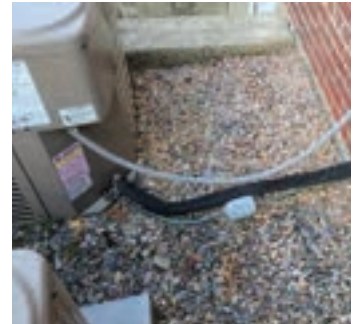
Photo 28: View of typical refrigerant piping from CUs
