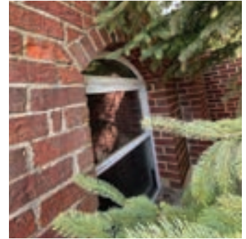
Photo 6: Planting conflict with building materials
