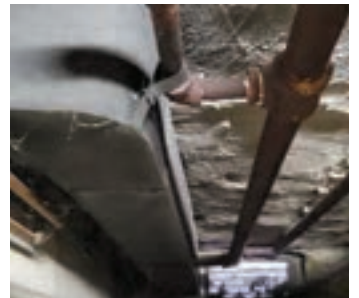
Photo 29: Combustion air louver
