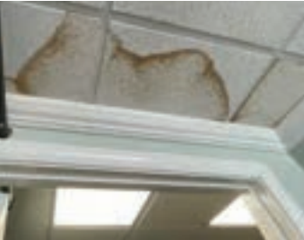
View of water damage on ACT tiles
