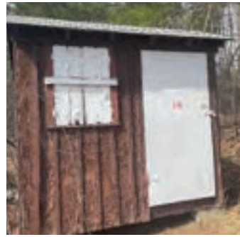
Photo 14: Painting peeling and wood rotting
