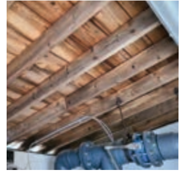
Photo 24: Pump house building interior
